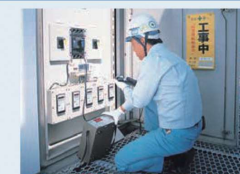
遮断器定期点検 Periodical inspection
