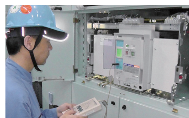
過電流保護装置の動作確認 Testing operation of over current protection devices
