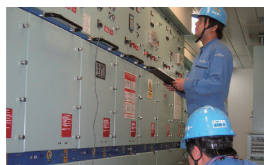
高圧配電盤復電前の安全確認 Safety check of high voltage plant prior to restoring power
